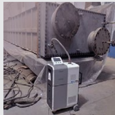
Heat exchanger detection
