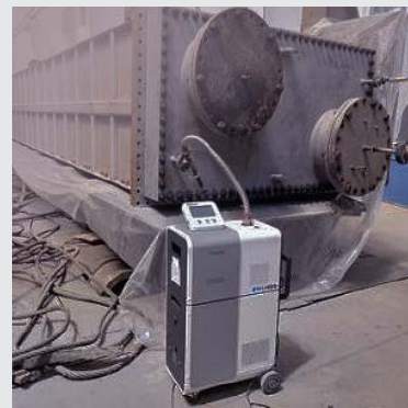
Heat exchanger detection
